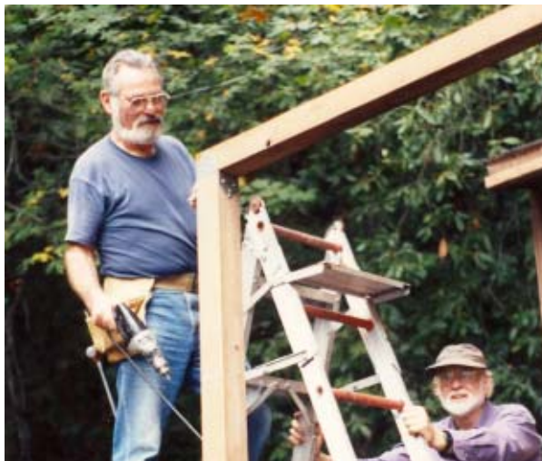
Bill Lipton on the ladder and Russ Whitman working on the deck roof at the Armstrong VC in about 1993.
